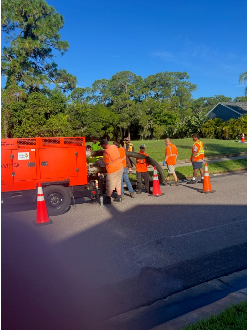
Pinellas County workers setting up pump station on Toniwood Ln that pumps water from the street and into ponds on Tarpon Woods Golf Course on 08/29/2024 after during a period of unseasonal exceptionally hard rain not tied with any tropical system. The same rain flooded several streets the day before.
